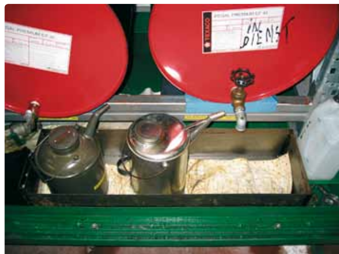
OP pads under oil cans & drums to catch small drips.
